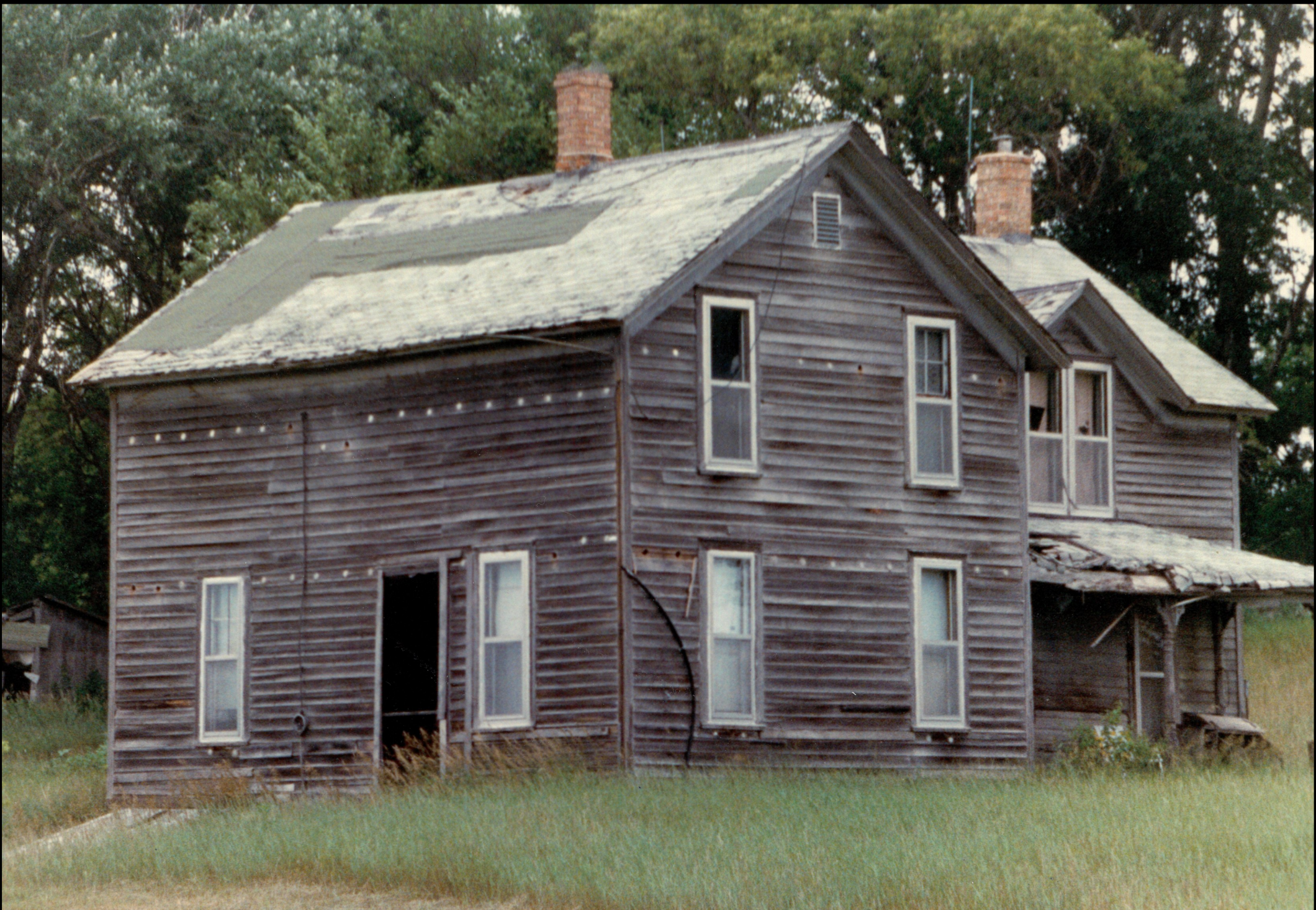
All that remains of the original house is the stone foundation. No well for a water supply was ever needed as spring water was piped directly into the basement. Above: Picture is the east and south sides of the house. Below: is the west and north sides of the house.
